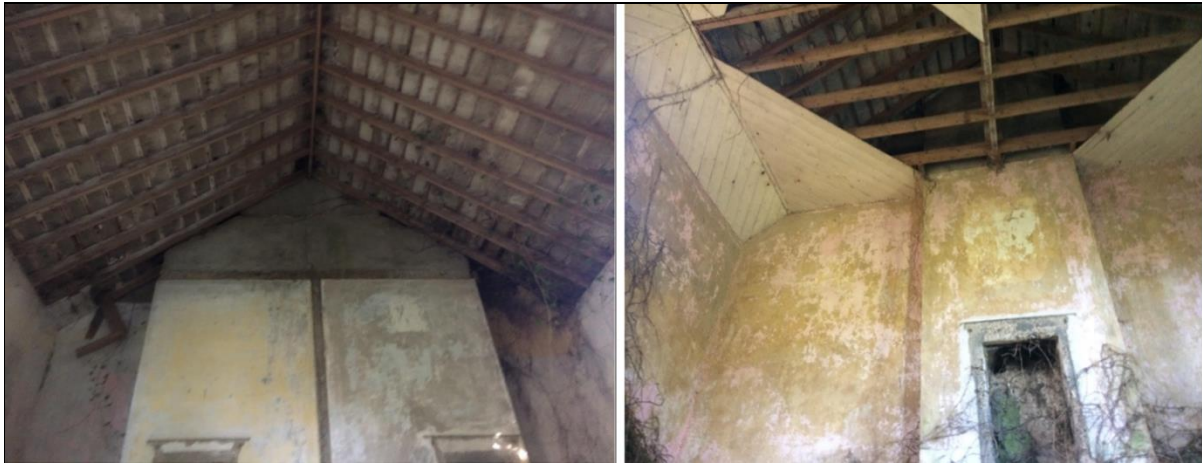
Photographs 5 – 6: Internal structure of building along with exposed roof beams and small sections of wooden cladding.
